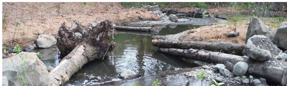
Example of natural materials (fallen tree, rootwad, boulders, logs, etc.) used in restoration to improve fish & wildlife habitat
