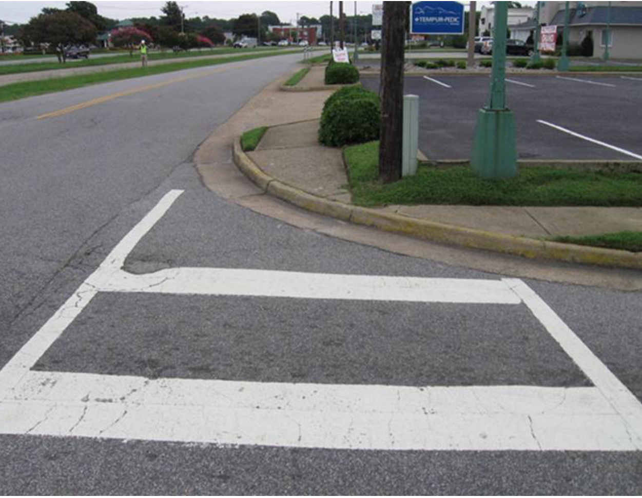
Absence of Curb Ramp
