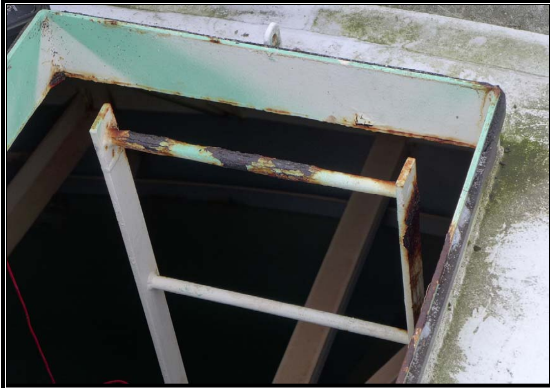
Photograph 5: 0.5MG Reservoir Hatch and Interior Ladder with Minor Corrosion
