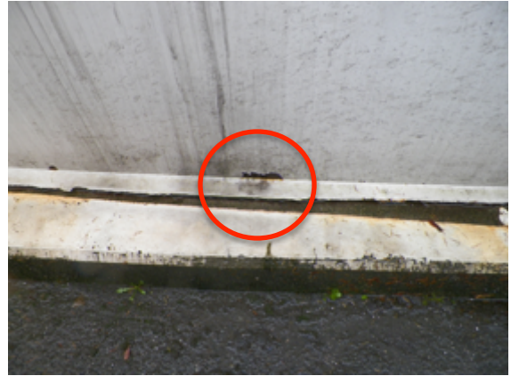
2.2 MG – Coating failure at chine
