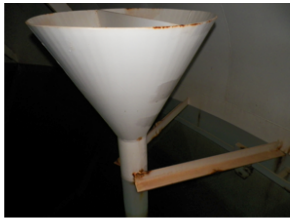
0.5 MG – Overflow pipe
