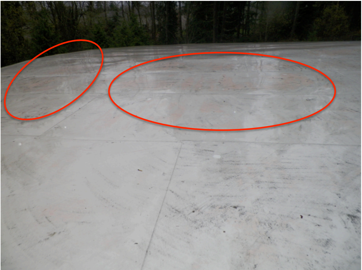
2.2 MG – Topcoat failure, comprising approximately 35 – 40% of roof
