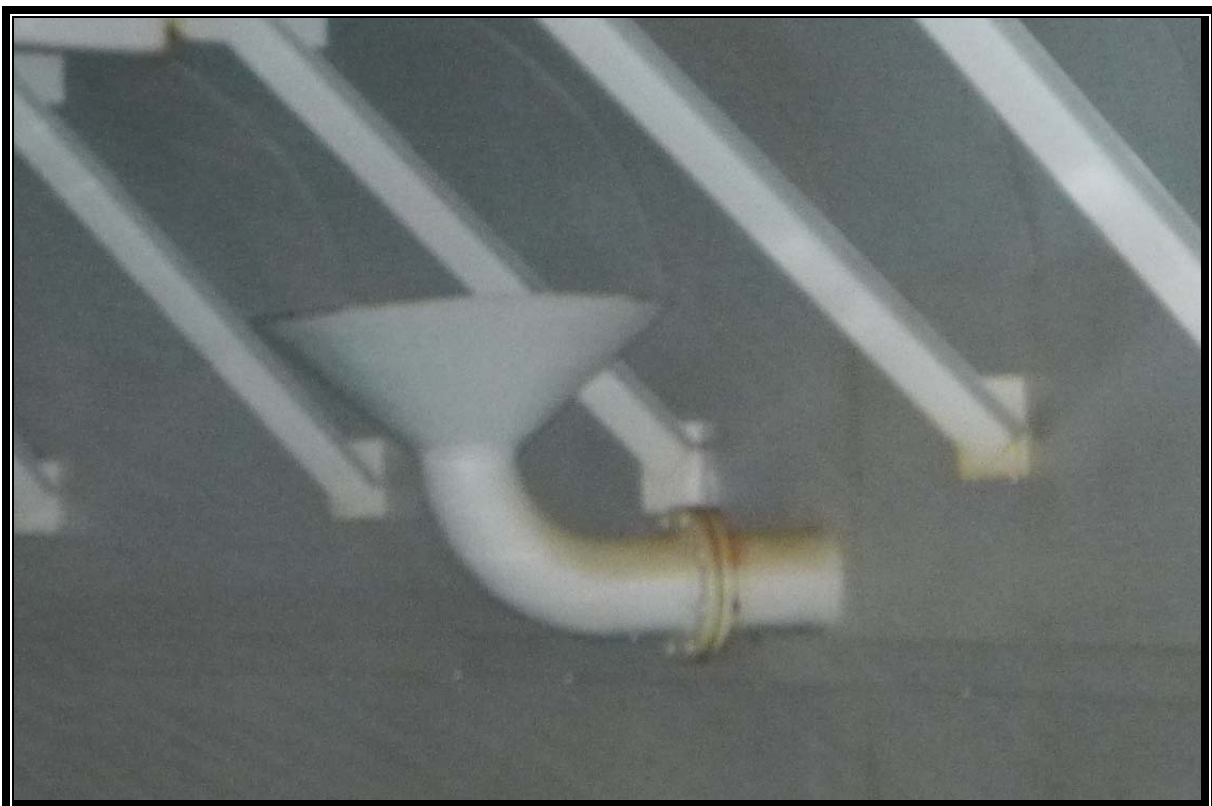
Photograph 18: 2.2MG Reservoir Overflow Pipe
