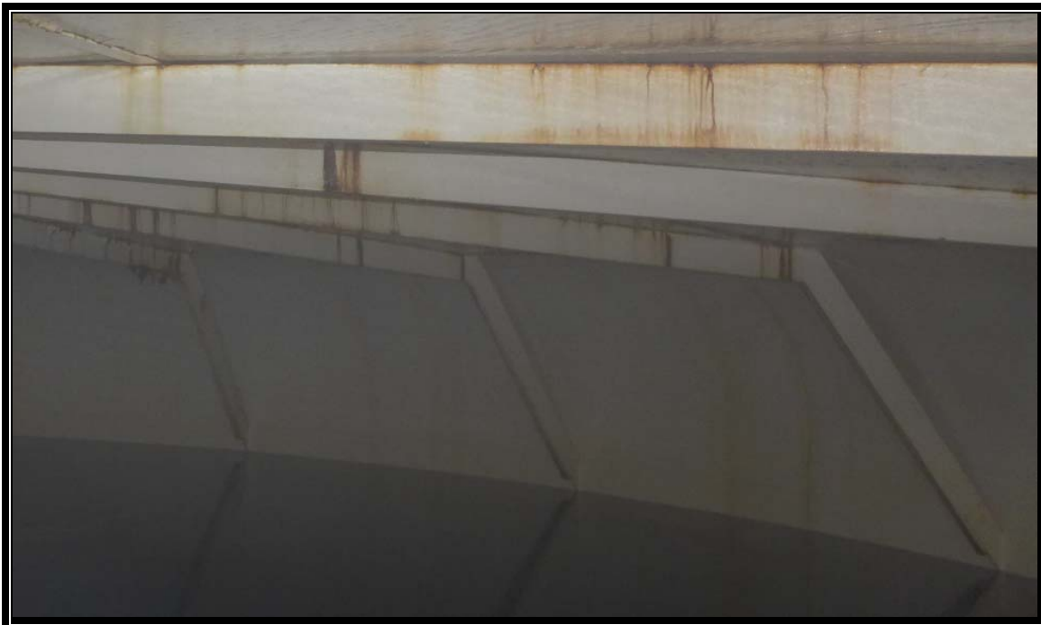
Photograph 10: 0.5MG Reservoir Corrosion of Roof Framing Members
