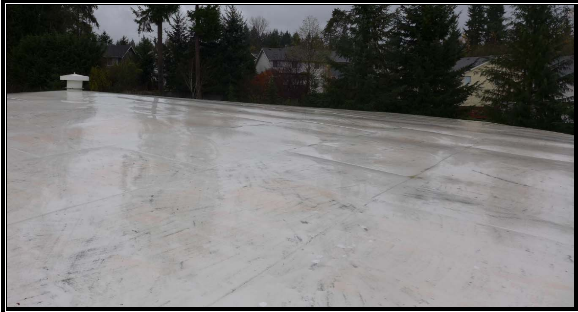
Photograph 13: 2.2MG Reservoir Buckled Roof Plates
