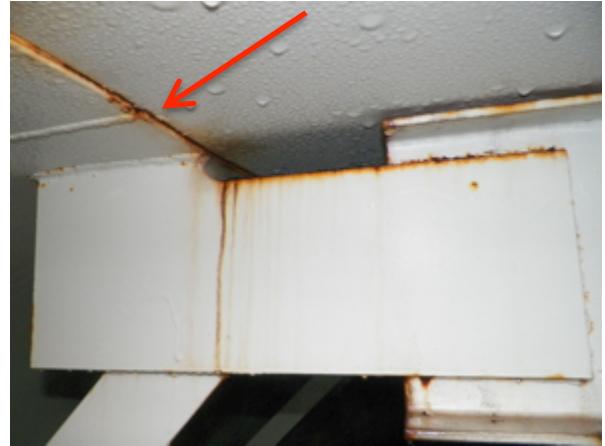
2.2 MG – Interior roof and beam overlaps with crevice corrosion
