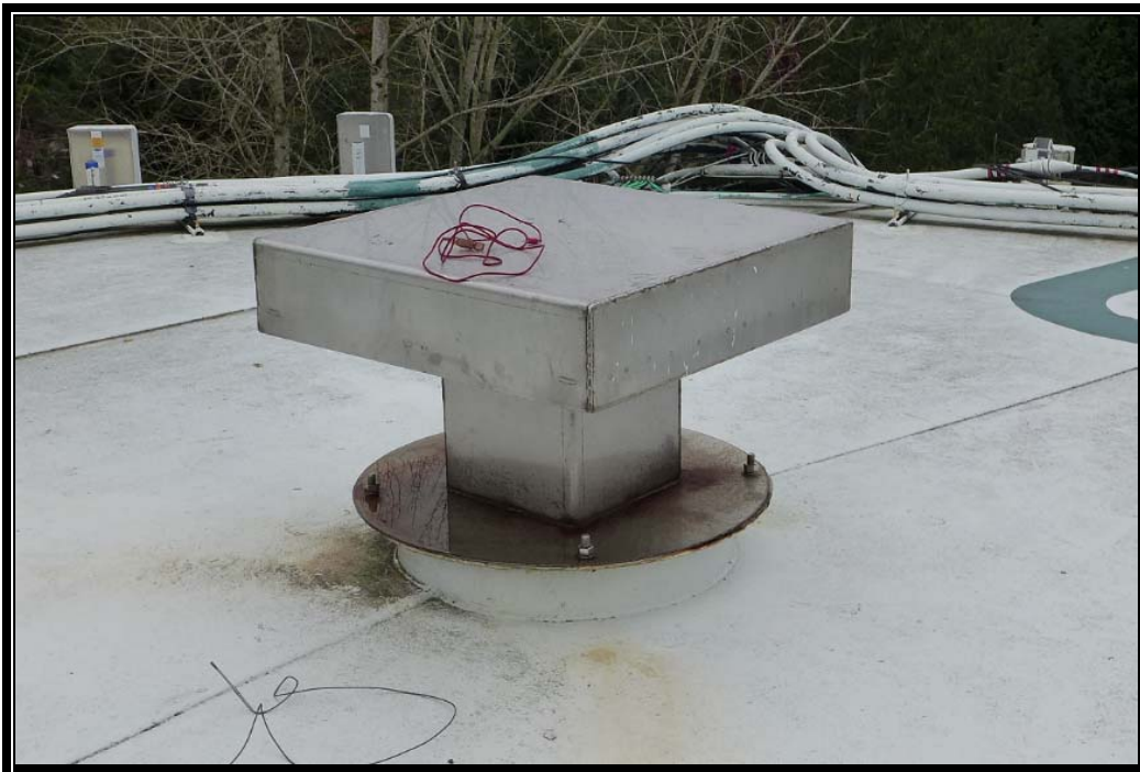
Photograph 4: 0.5MG Reservoir Vent
