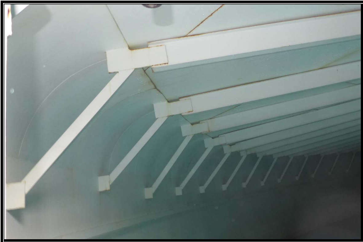
Photograph 16: 2.2MG Reservoir Roof Plates with Minor Corrosion
