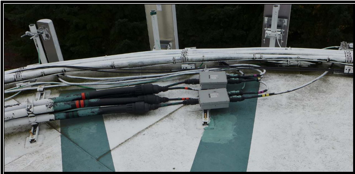
Photograph 6: 0.5MG Reservoir Cellular Transmission on Roof
