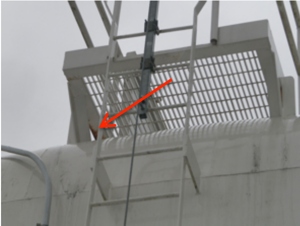
2.2 MG - Missed coating on bottom of exterior landing
