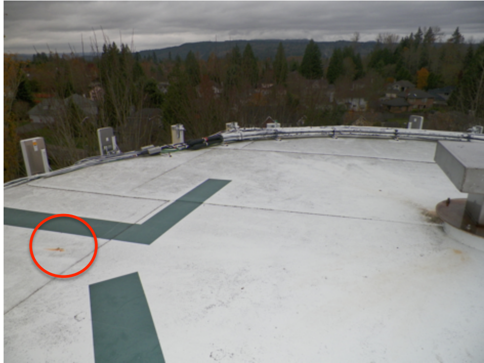
0.5 MG - Dirt on roof and small coating defect
