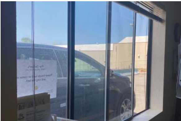
Windows throughout the building are un-insulated and may not be properly flashed.
