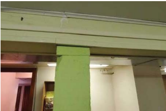
Lower level post is not anchored to the beam.
