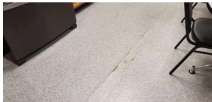
Cracks at the break room
