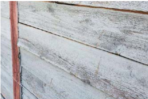
Detached siding at the east elevation
