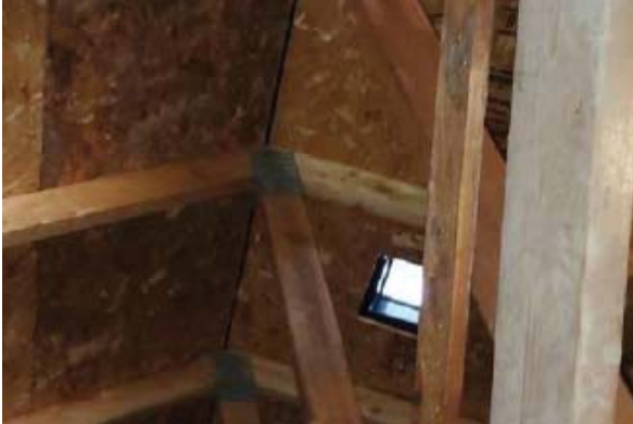
The roof structure consists of pre-manufactured plated wood trusses and are in good condition.
