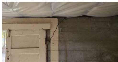
Cracks and signs of movement on the west wall
