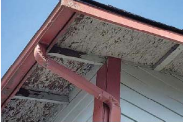
Paint is peeling and the OSB roof sheathing is exposed. Prolonged exposure can cause the sheathing to swell and deteriorate.
