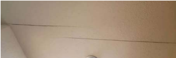
Transition cracks at the ceiling.
