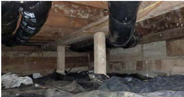
Top: Farmhouse floor framing around chimney and damaged joists. Bottom: Farmhouse crawlspace posts without anchorage.
