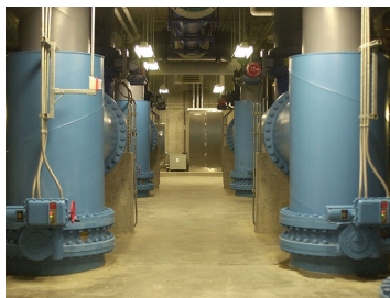
The interior of the Tolt water treatment facility . Photo Credit SPU
